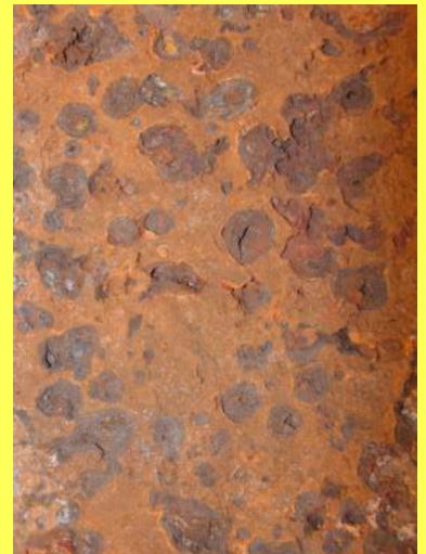
Localised corrosion for high levels of salt
