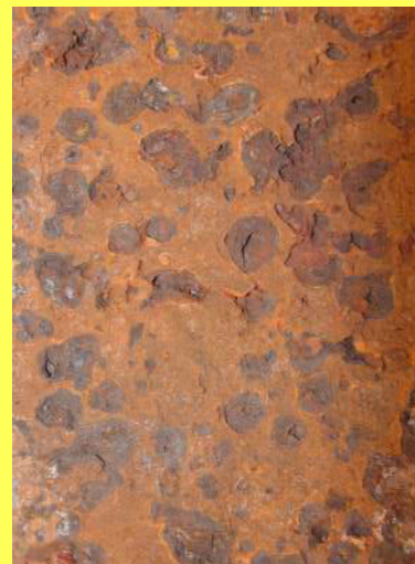
Localised corrosion for high levels of salt
